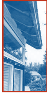
Open eaves, vents not screened (6 pts)
